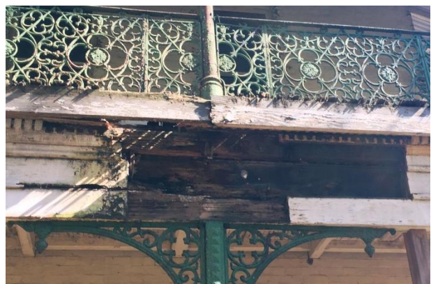
Timber damage on the exterior wooden balcony
